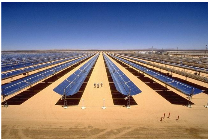
Figure 4. Parabolic power plant in the Mojave desert in California (source: DESERTEC-UK ).
