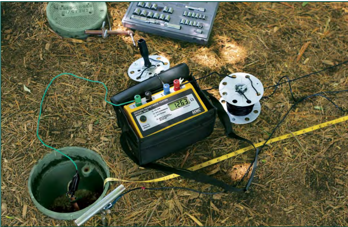
Ground Resistance Tester Model 4610 checks the ground rod using the Fall-of-Potential method.
