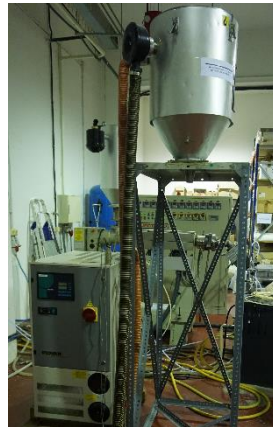
Figure 7. PIOVAN desiccant dryer for PLA and REX-PLA extrusion.
