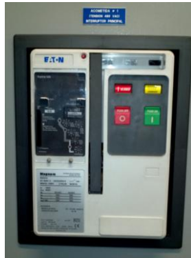
Figura 12: Interruptor principal Acometida 1
