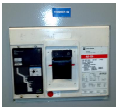
Figura 16: Transfer del tablero principal 02 (TP-02)
