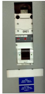
Figura 52: interruptor By-Pass UPS 2.2.
