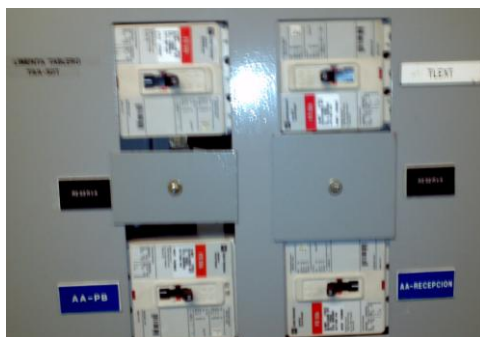
Figura 15: Interruptor del tablero principal 02 (TP-02)
