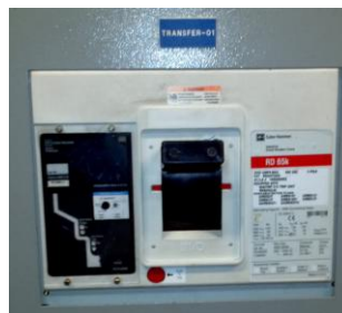
Figura 11: Transfer del tablero principal 01 (TP-01)
