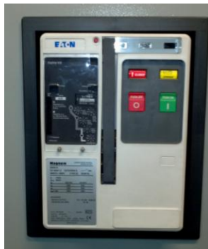
Figura 21: Interruptor acometida 1 del interruptor TPTC.
