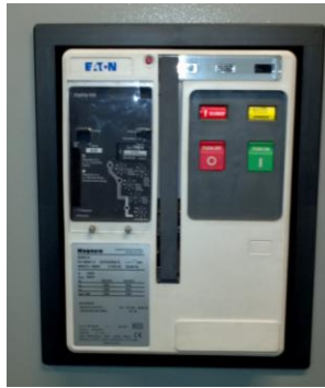
Figura 25: Interruptor acometida 2 del interruptor TPTC.
