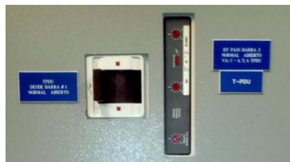
Figura 51: Interruptor By-Pass UPS 2.2.
