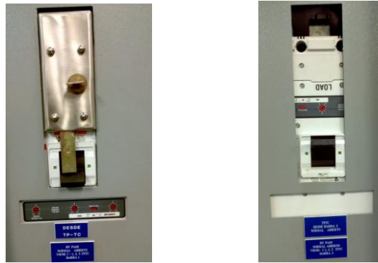
Figura 45: interruptor By-Pass UPS 2.1.
