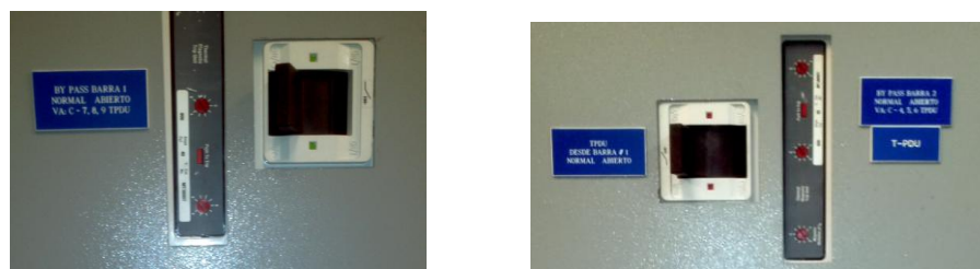
Figura 44: Interruptor By-Pass UPS 2.1.
