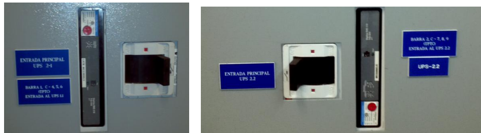
Figura 42: Interruptor principal de UPS 2.1.
