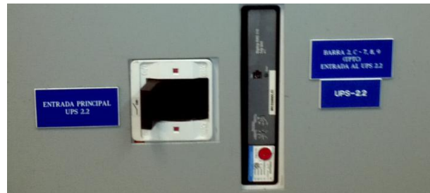
Figura 49: Interruptor principal de UPS 2.2.
