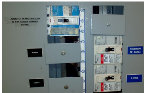
Figura 10: Interruptor del tablero principal 01 (TP-01)
