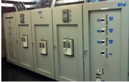
Figura 18: Tablero de Transferencia (TPTC).
