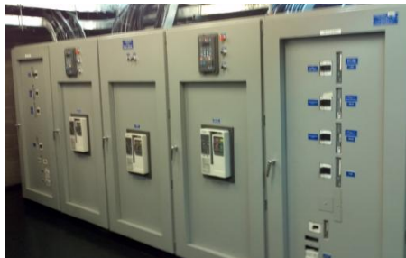
Figura 22: Tablero de Transferencia (TPTC)
