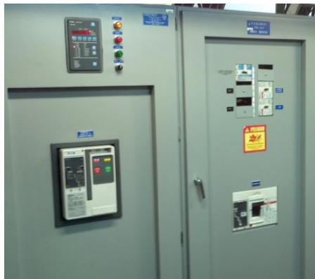
Figura 8: Tablero Principal 01 (TP-01)
