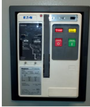
Figura 17: Interruptor principal acometida 2
