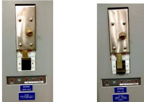
Figura 33: Interruptor salida UPS 2.2 e interruptor de BY-PASS.
