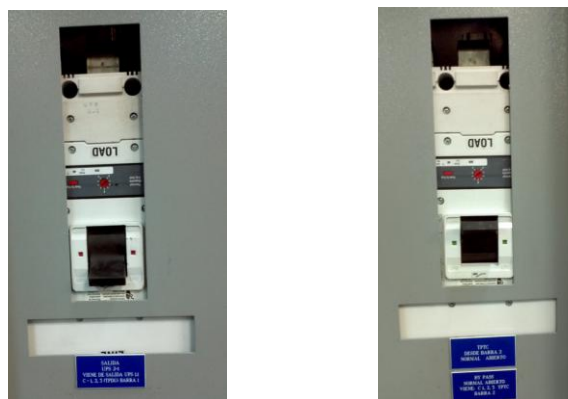
Figura 30: Interruptor salida UPS 2.1 e interruptor de BY-PASS.
