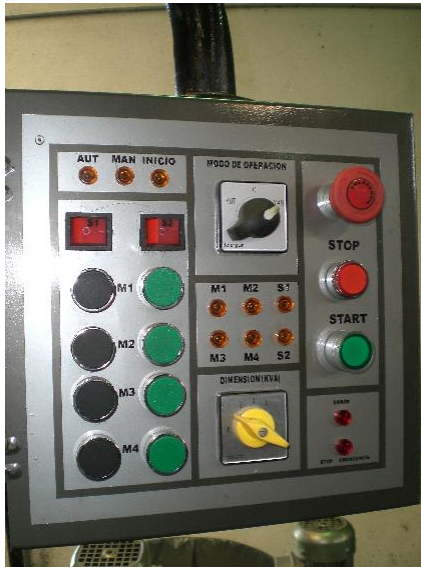
Figura N27. Panel de Control
