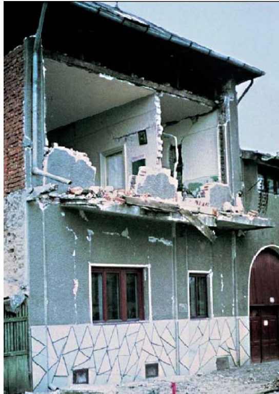
FIG. 9.3. Desprendimiento de paredes (Seismic Conceptual Design of Buildings. Hugo Bachmann)
